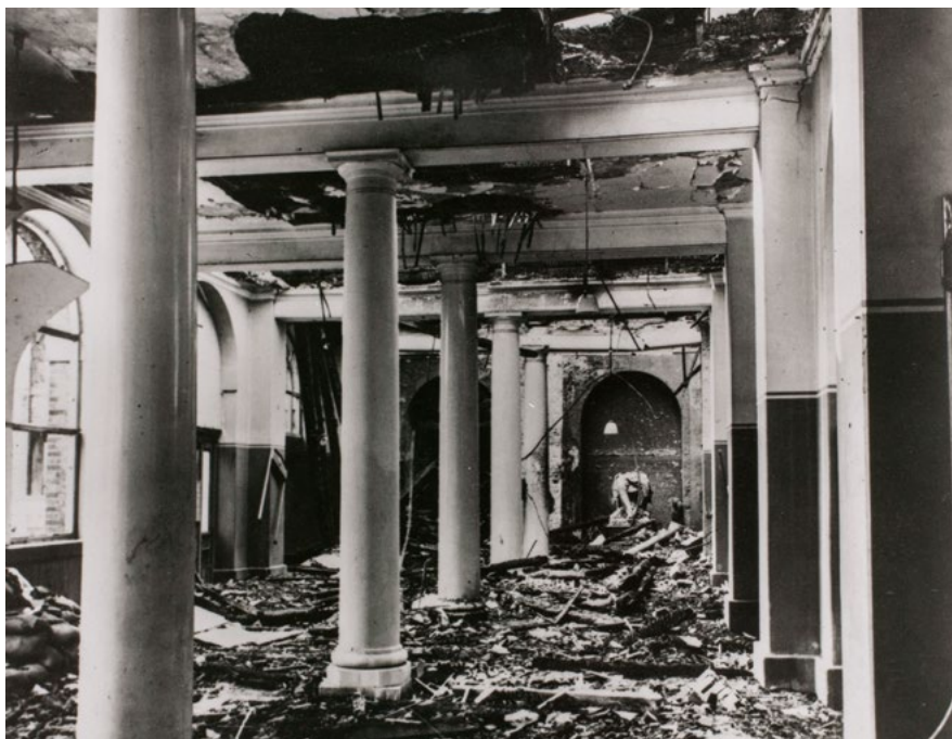
Second World War bomb damage at UCL, including the destruction of the Great Hall and parts of the main building's cloisters. UCL Special Collections.
