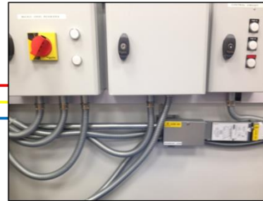
415 V AC Microgrid
