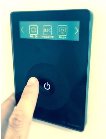
Figure 9: Lighting for the room is controlled by the intuitive touch-wheel and touchscreen unit allowing users to select pre-set scenes optimised for particular areas and activities.
