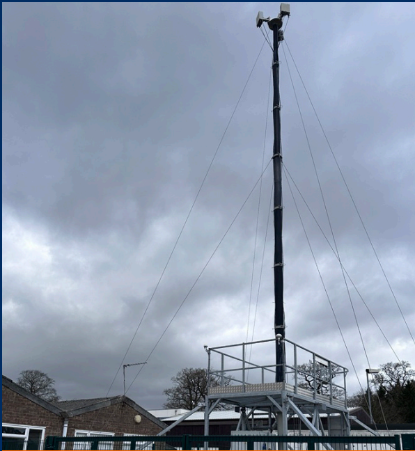
Mobile 5G-SA Mast
