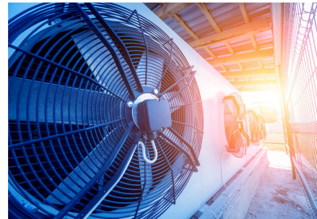
HVAC in commercial buildings
