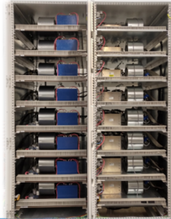
Power Module Cabinet
